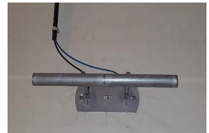
Pitot tube on opposite side and pneumatic connection to terminal box
